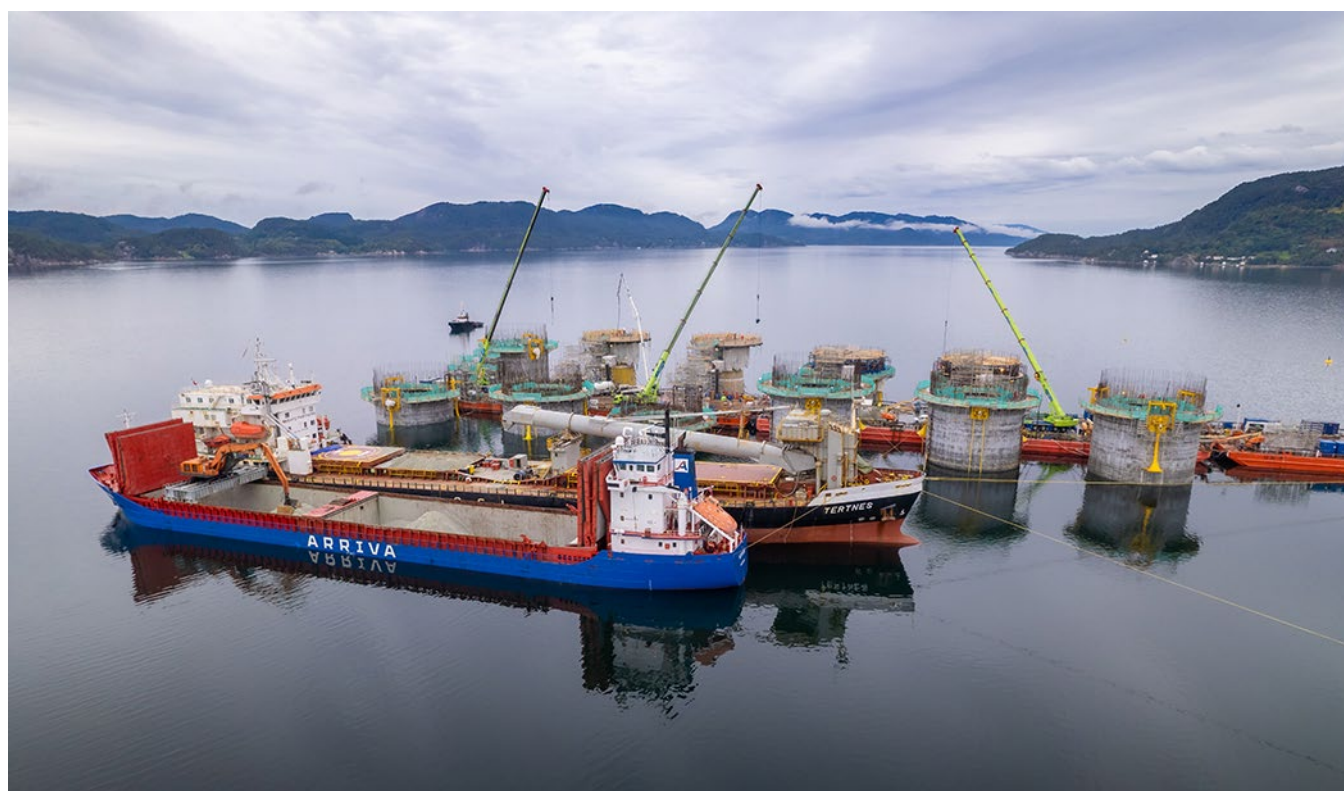
Slipforming at Dommersnes in July 2021, of substructures for Hywind Tampen floating offshore wind farm.
